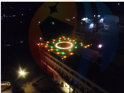
Heliport Lighting on roof of building
